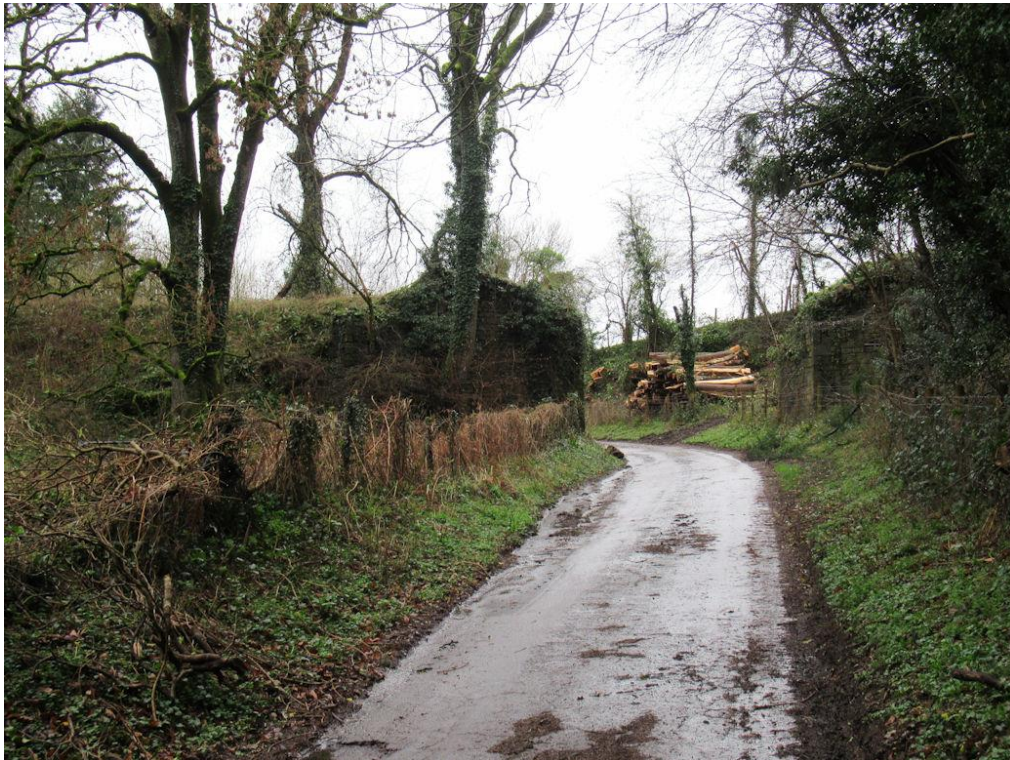
By 2024, the railway bridge survives in reasonably good condition. The survival prospects of the tramway bridge have been improved by removal of trees and vegetation.
