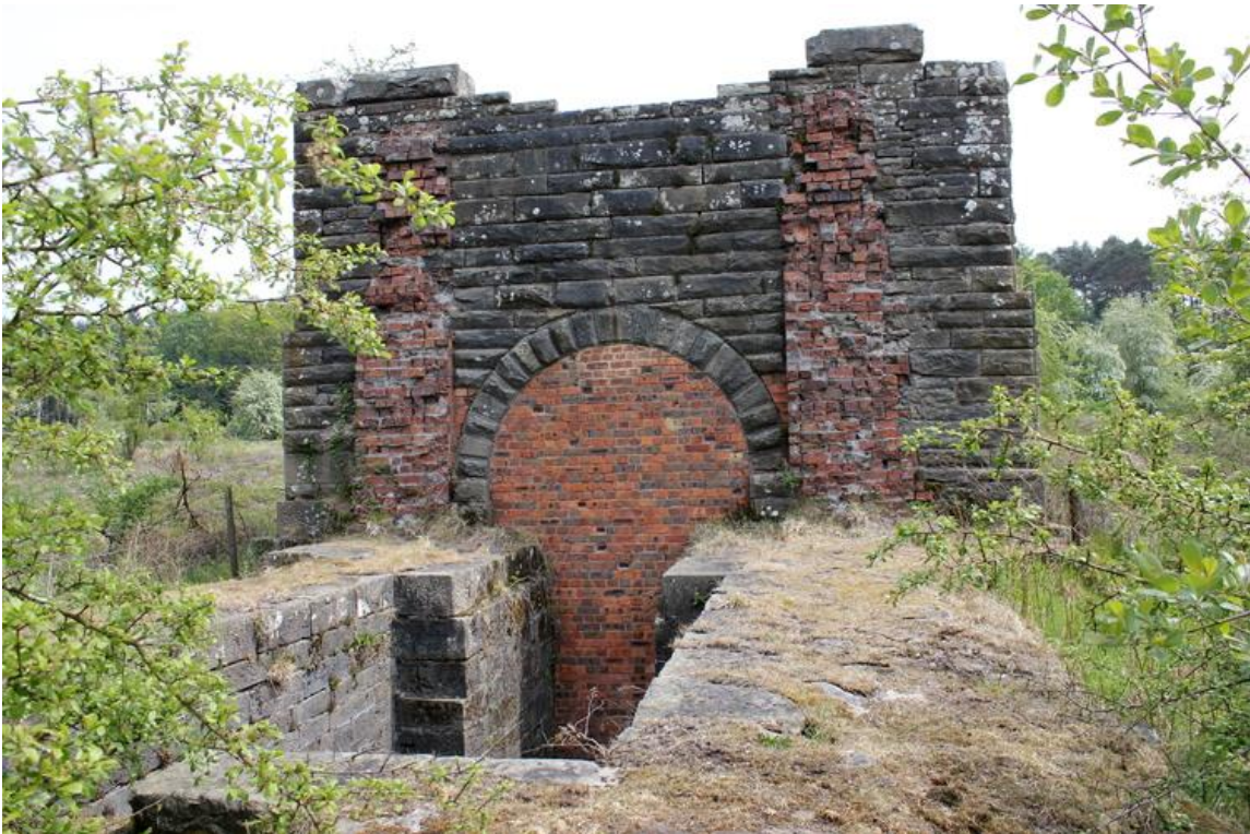
Clearance of the surrounding vegetation has made the remains of the old engine house more visible.
