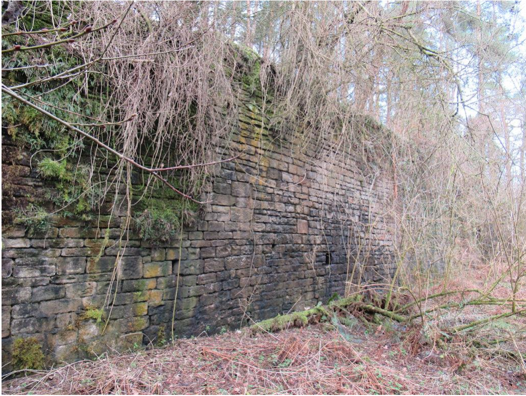
Evidently Forestry England have been conserving the screens to some extent, as evidenced in vegetation removal and limited repointing of the wall
