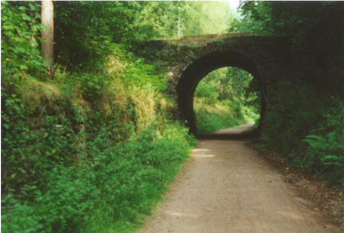
Trafalgar Arch, near Brierley - Bridge over the former Severn and Wye Railway. The bridge carried colliery 'traffic' and renovated when the former railway track was incorporated into a family cycleway.
