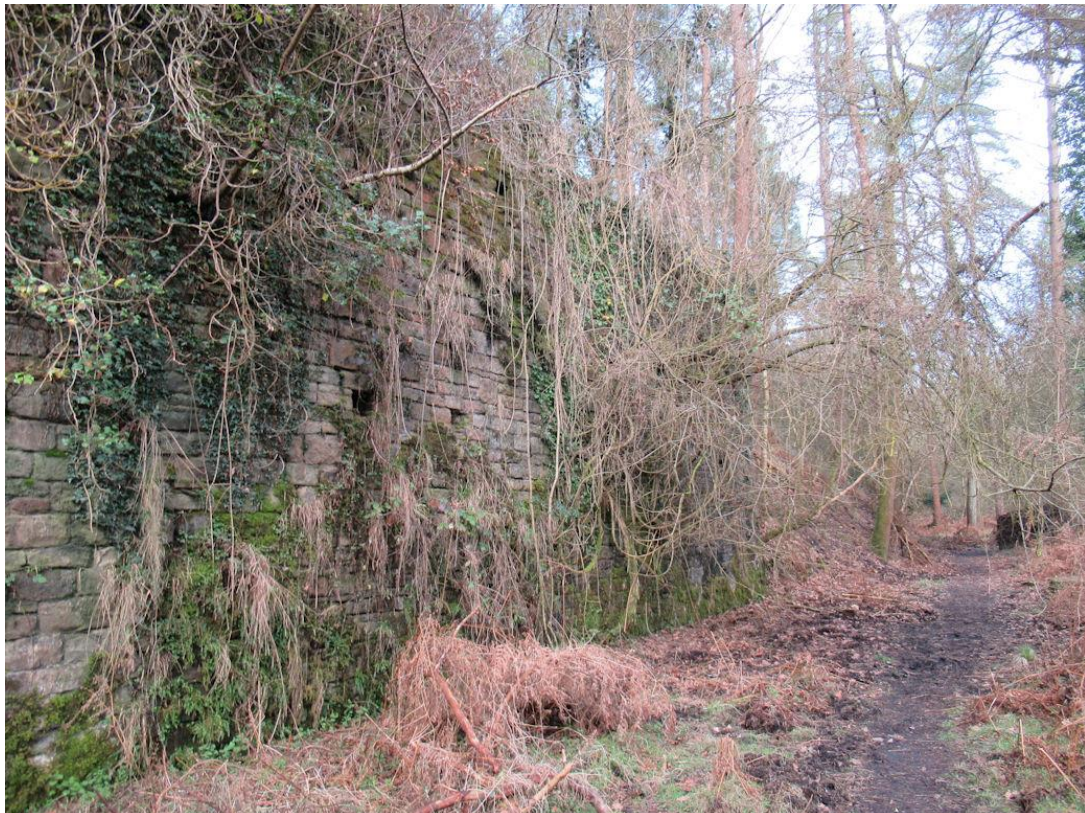
However, there are still a few trees rooted in some sections of the wall
